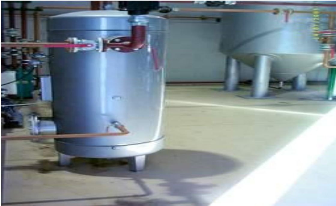
Figure (4.3): pneumatic tanks
