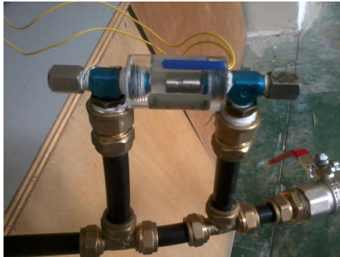
Figure(6.4) : Flow Sensor Connection
