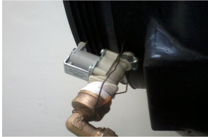
Figure(6.13): Electric Valve
