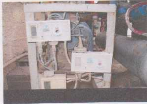
Figure (3-9) Pressure and Temperature Controls and Refrigerant Accumulator
