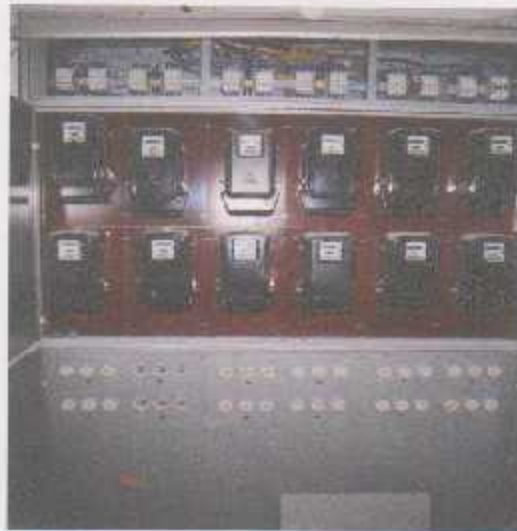
Figure (3-16) Electrical Cabinet of Station
