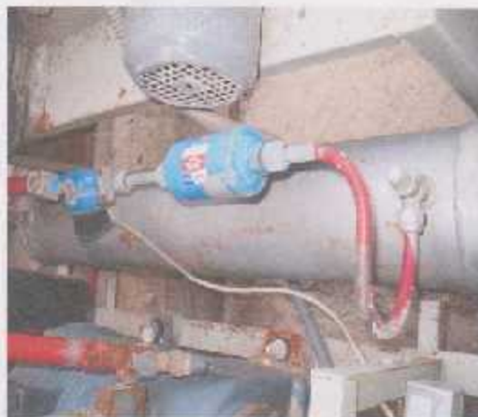
Figure (3-8) Filter Dryer and Solenoid Valve
