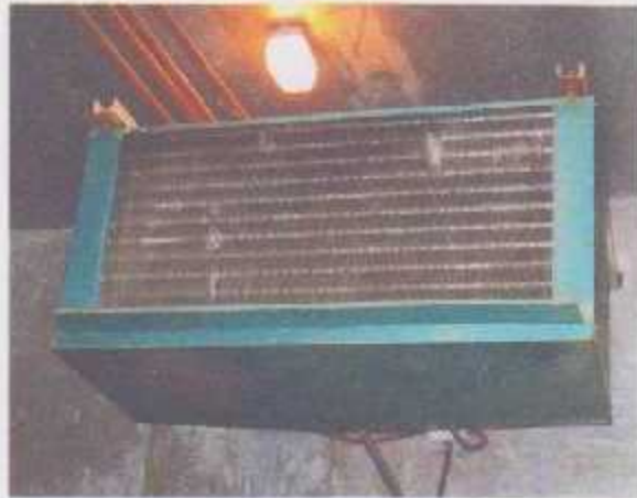
Figure (3-5). Indoor Evaporator
