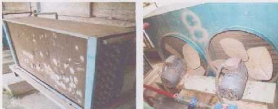
Figure (3-6). Outdoor Condenser
