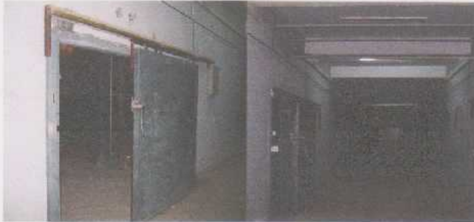
Figure (3-1).Photos Taken inside the Refrigeration Station
