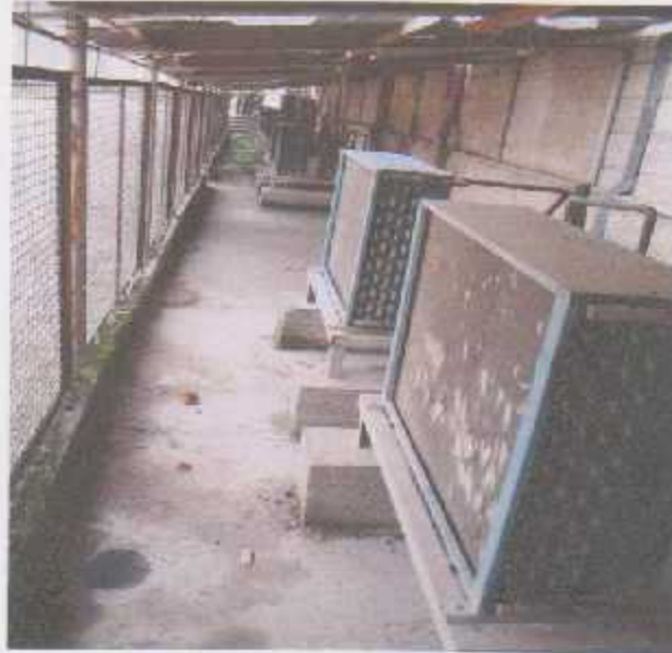
Figure (3-15) Outside View of Outdoor Refrigeration Units
