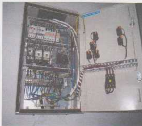
Figure (3-17) Control Cabinet for each Room
