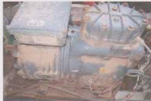
Figure (3-4) Compressor Used in the Station
