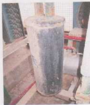
Figure (3-10) Oil Separator
