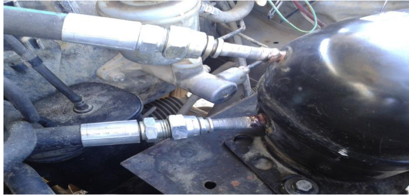
Figure 4.14: Compressor Cooling with pipe connector.
