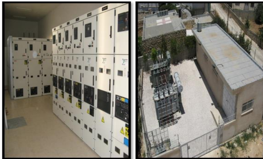
Figure (2.10): Power Transformer and switchgear in Alhusein substation.
