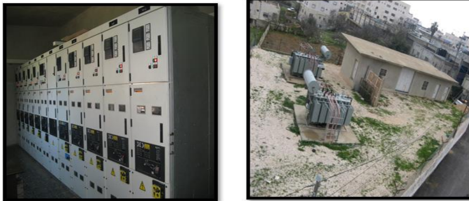
Figure (2.14): Power Transformer and switchgear in Alduhdah substation.
