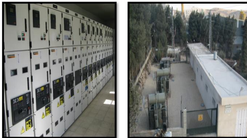
Fig. (2.2): Power Transformer and switchgear in Alfahas substation.
