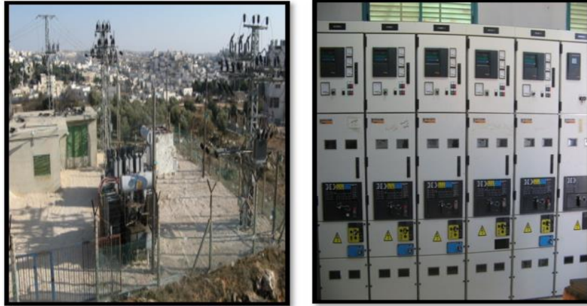
Figure (2.12): Power Transformer and switchgear in Alras substation.
