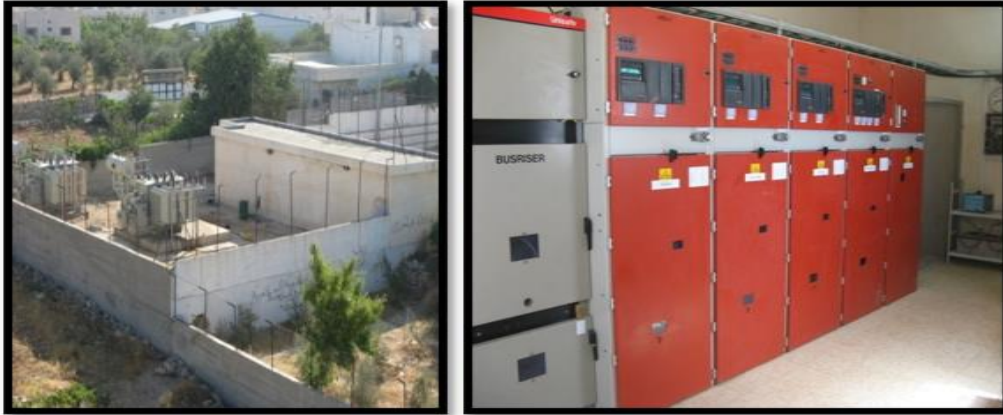
Figure (2.8): Power Transformer and switchgear in Alhareaq substation.
