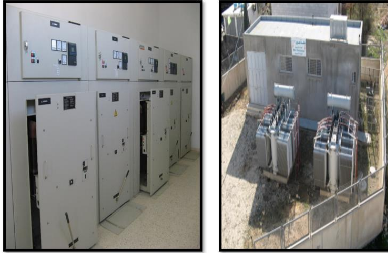
Fig. (2.4): Power Transformer and switchgear in West substation.
