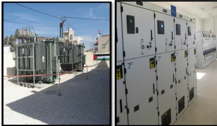
Fig. (2.6): Power Transformer and switchgear in Umaldaleh substation.
