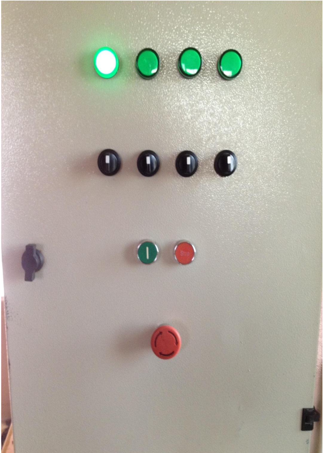
Figure (6.6): Actual panel electric from outside.
