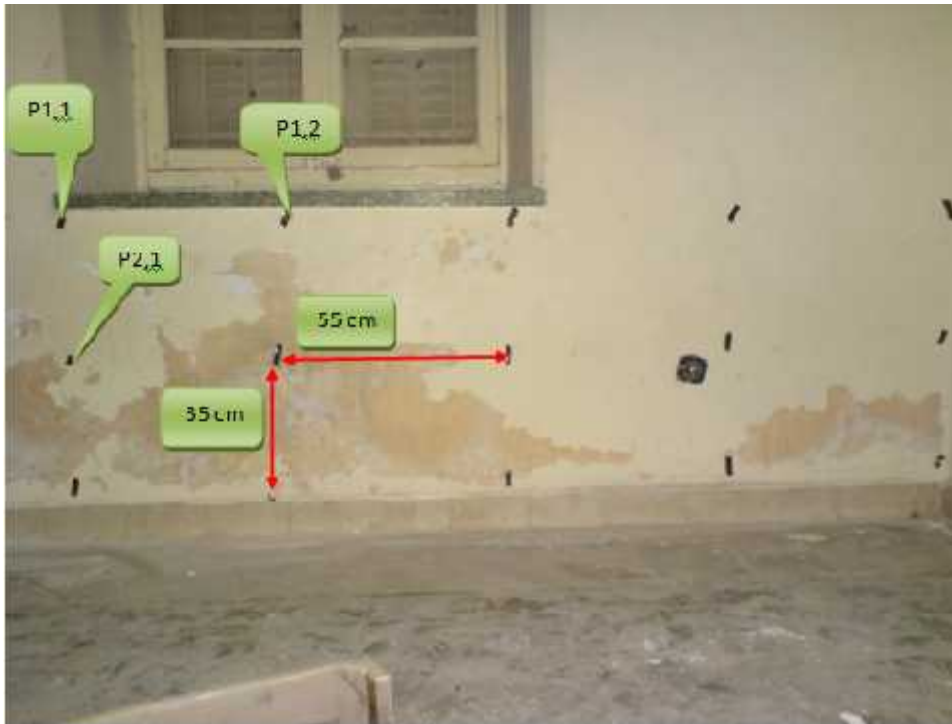
Figure 4.13: the distribution of points at the inner side of wall in class 2.
