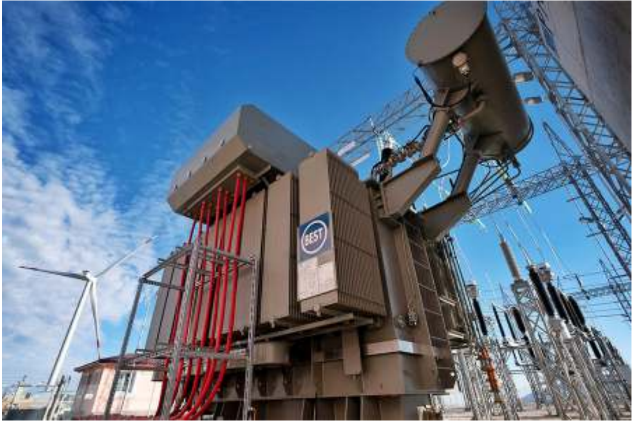
Figure 3 Transformers used in the station.
