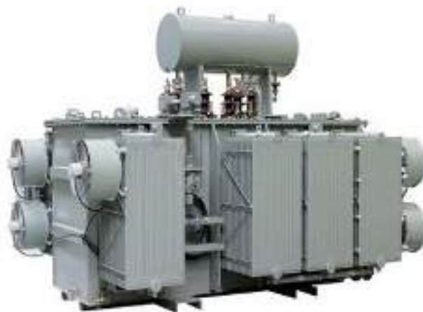
Figure 2Minera MP Schneider power transformer
