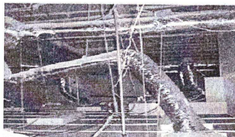
Figure(4-2) Air ducts
