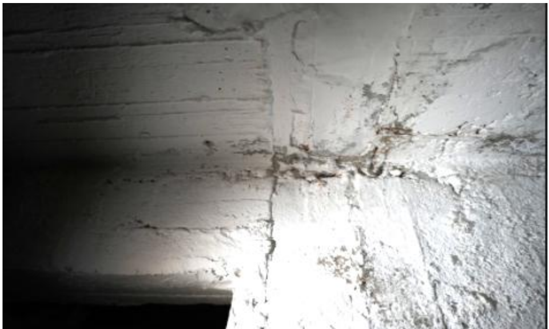
Figure 4.3: Localized cracking, moisture-related deterioration, and minor reinforcement corrosion observed in a reinforced concrete connection region during the field assessment.
