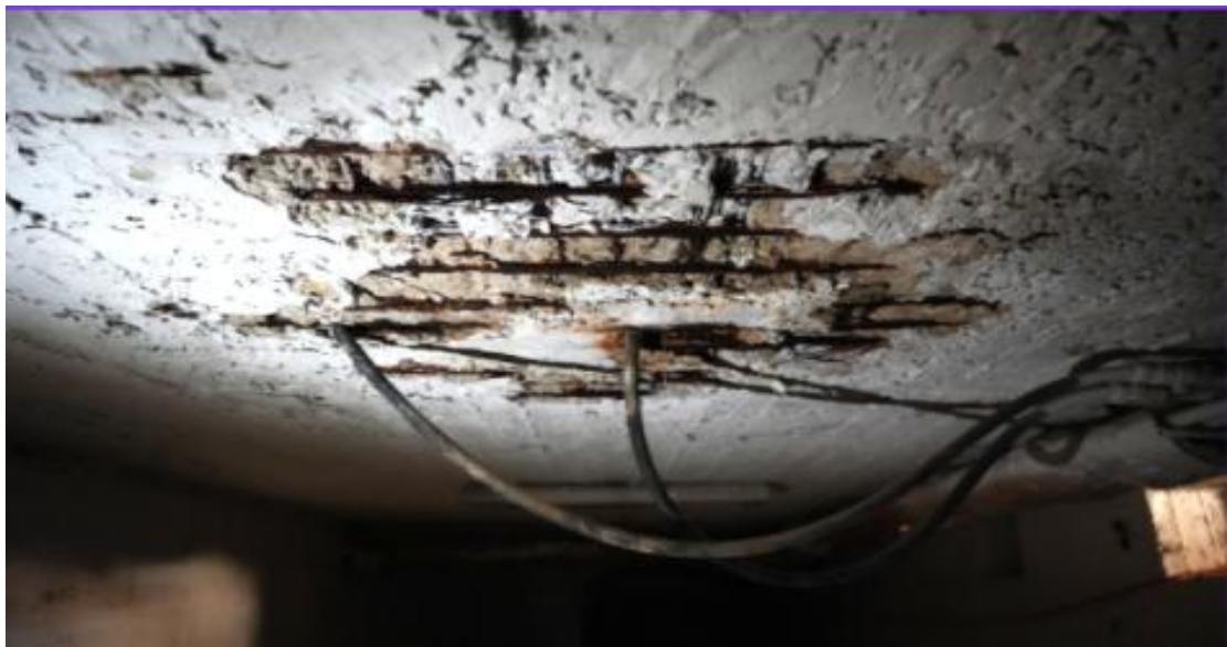
Figure 4.5: Localized reinforcement corrosion and concrete cover deterioration observed in an existing reinforced concrete slab during the field inspection.
