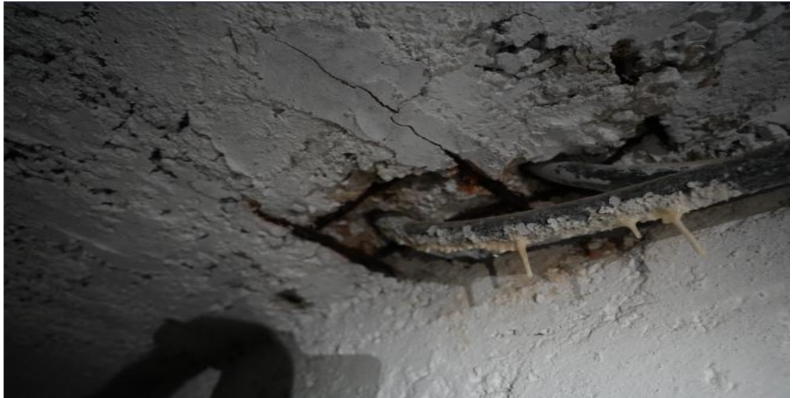
Figure 4.4: Deterioration of reinforced concrete characterized by reinforcement corrosion, cracking, and loss of concrete cover in a weather-exposed structural element.
