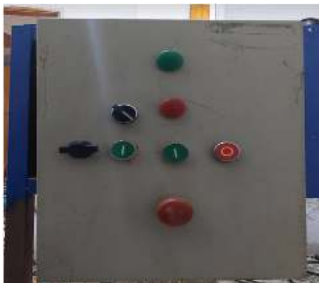
Figure 5.4: Control panel (outward appearance)
