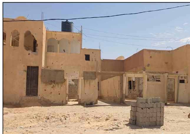
Figure 6. Some damaged houses
