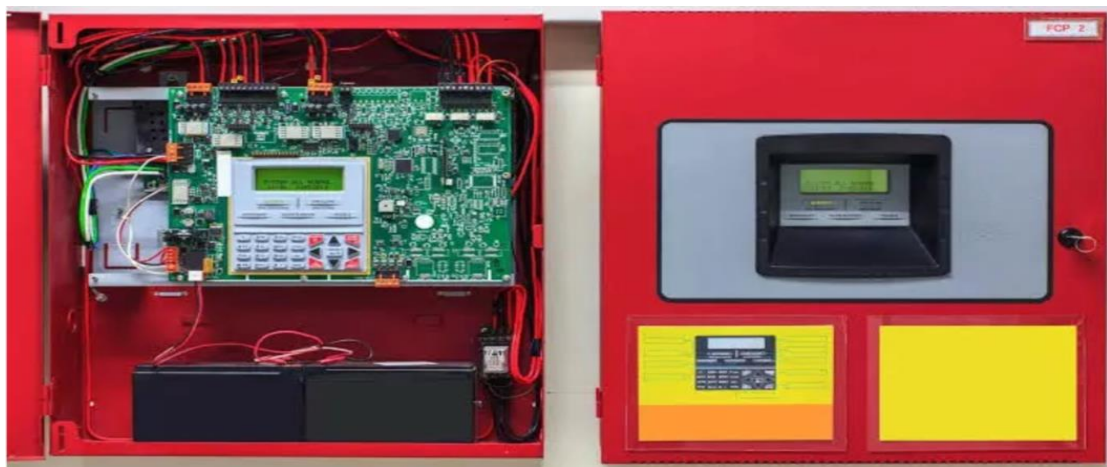
Figure 6.5 Fire Alarm Control Panel.[10]
