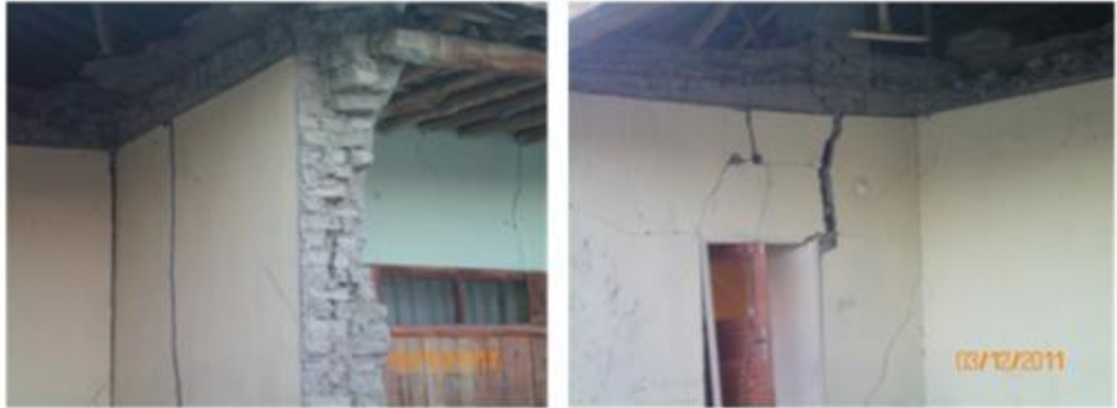
Figure 2.6: Inside view of shear cracking on structural walls in Turkey (Bayraktar, A., Altunışık, A.C. and Muvafık, M., 2016.) [3]
