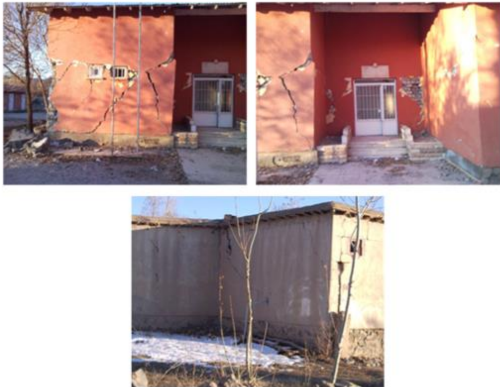
Figure 2.5: Outside view of shear cracking on structural walls in Turkey
