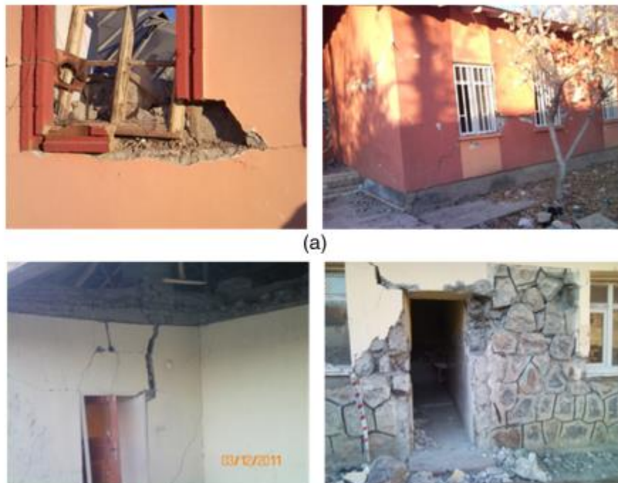
Figure 2.7: Cracks at corners of windows and doors in Turkey
