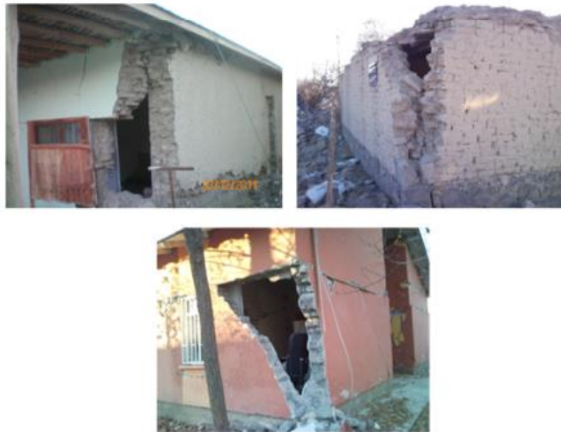
Figure 2.2: collapsed building corner at Edremit.
