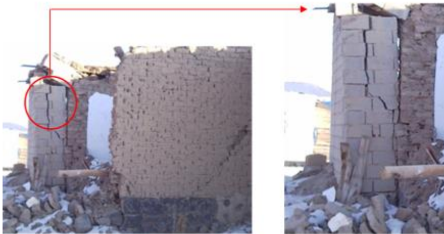
Figure 2.4: Failure of low-strength stone on a masonry building (Images by Alemdar Bayraktar) (Bayraktar, A., Altunışık, A.C. and Muvafık, M., 2016.) [3]
