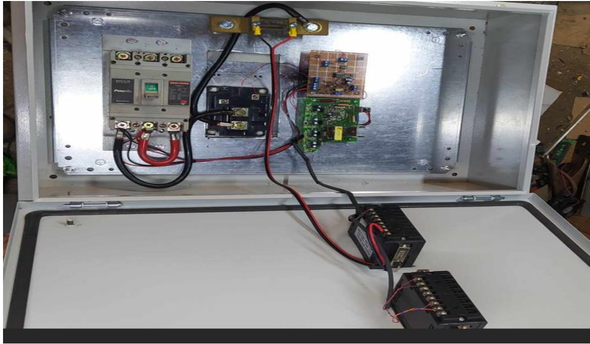
Figure13: Complete circuit assembly
