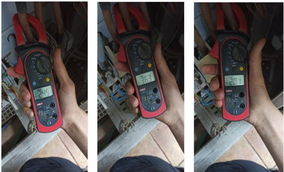
Figure14: Actual measurement of three-phase UPS current.
