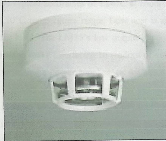
Figure (2.9): Fire Detector
