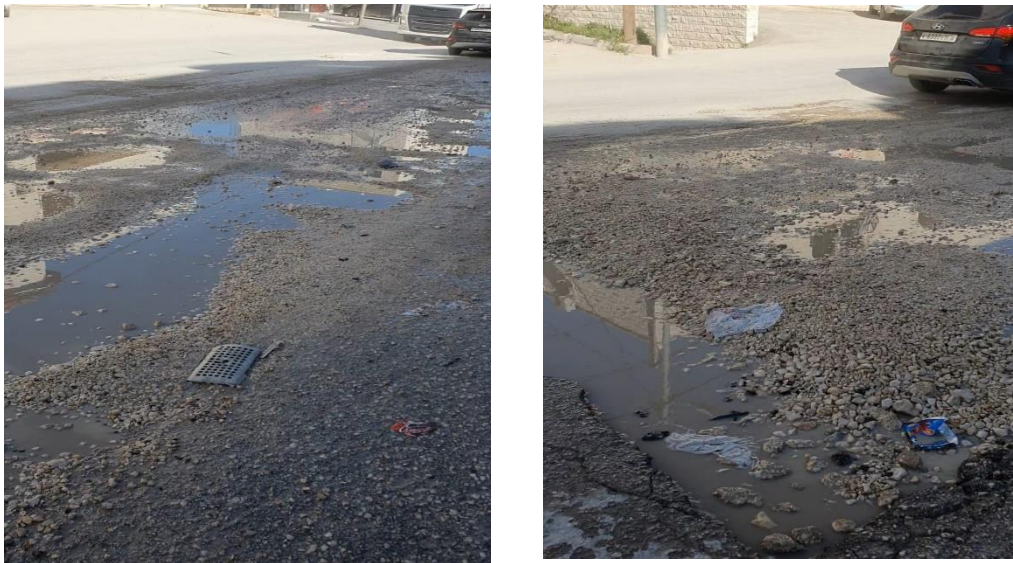
Figure 3.2: An image showing poor rainwater drainage
