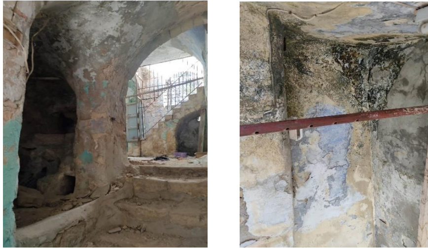
Figure 3.10: Mold inside of the building. Source: researcher
