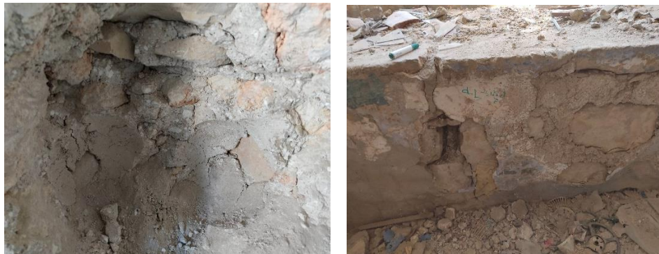
Figure 3.8: Fragmentation of the mortar between the stones. Source: researcher
