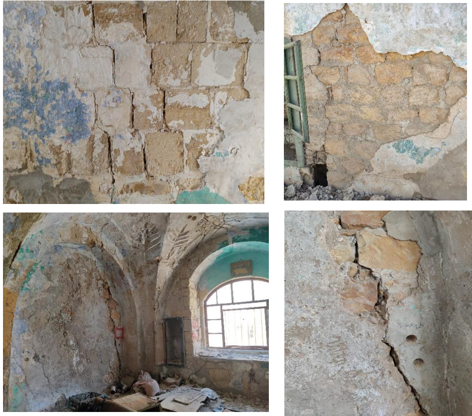
Figure 3.7: Different types of cracks of. Source: researcher
