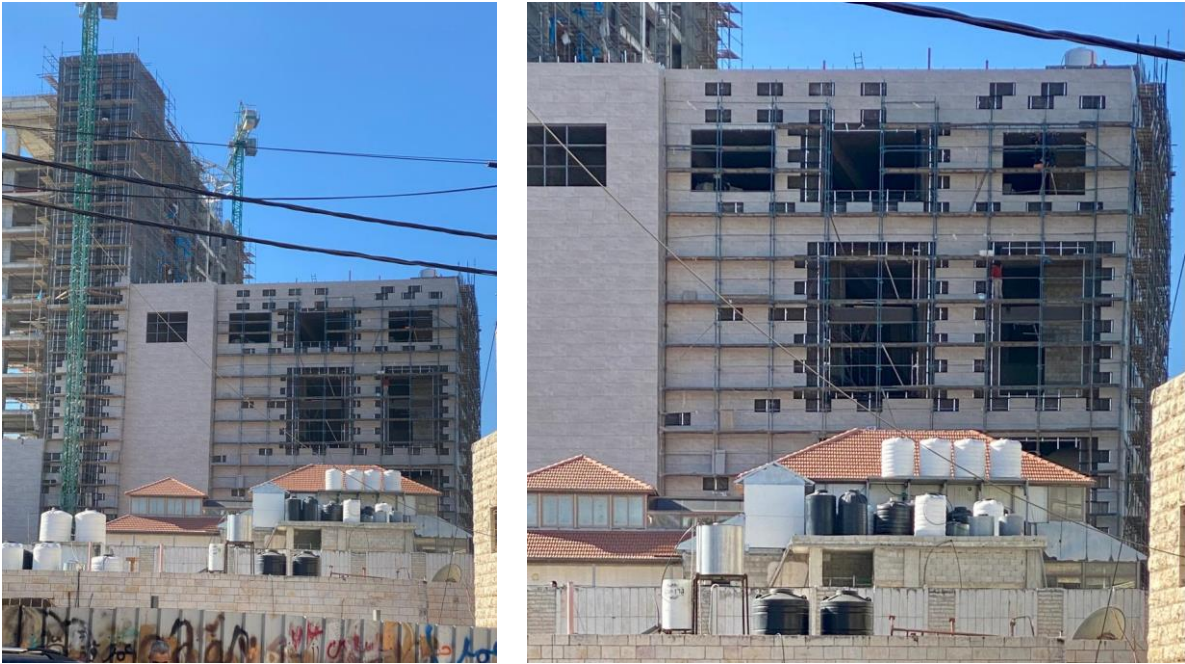
Figure 4-27 (b): Additional pictures for mechanical stone cladding on hollow concrete block walls in Hebron
