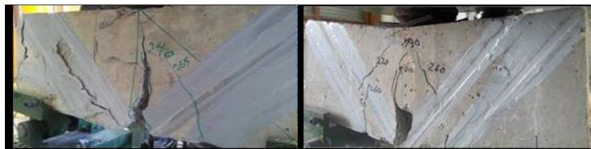
Figure 9 Adding CFRP rods to support shear to tested beams (Almassri et al., 2016)
