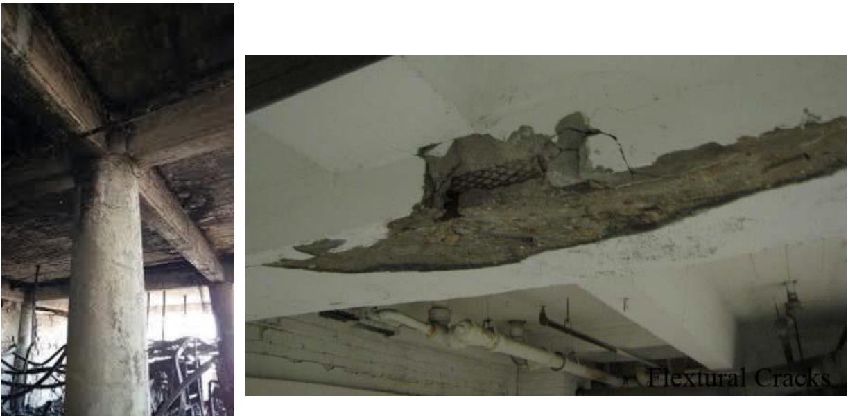
Figure 3 Structural Cracks and fire damages of RC buildings
