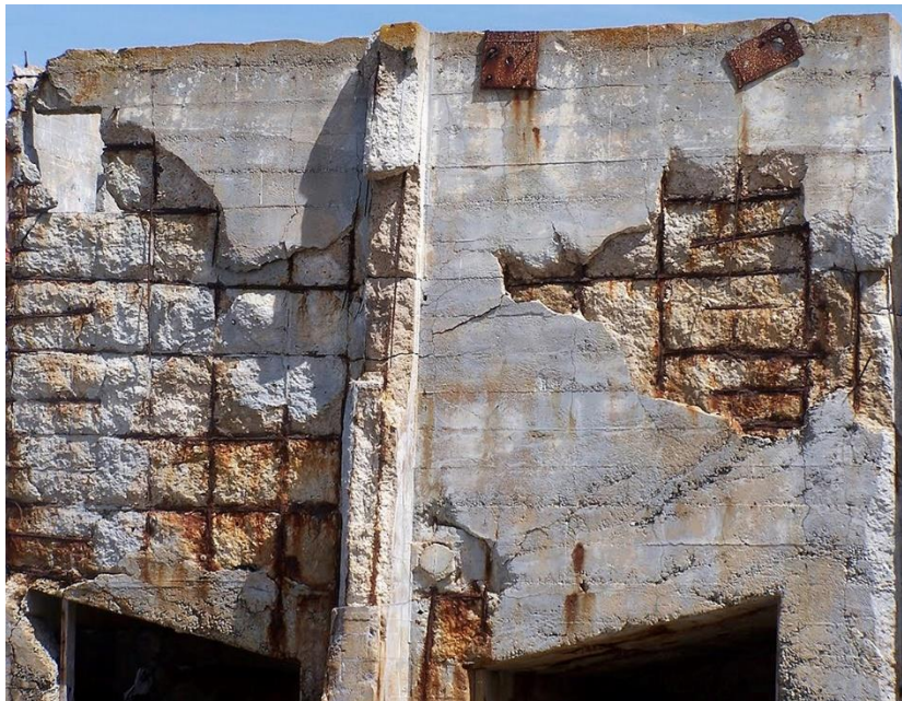
Figure 2 Reinforced Concrete Building with severe damage due to Corrosion
