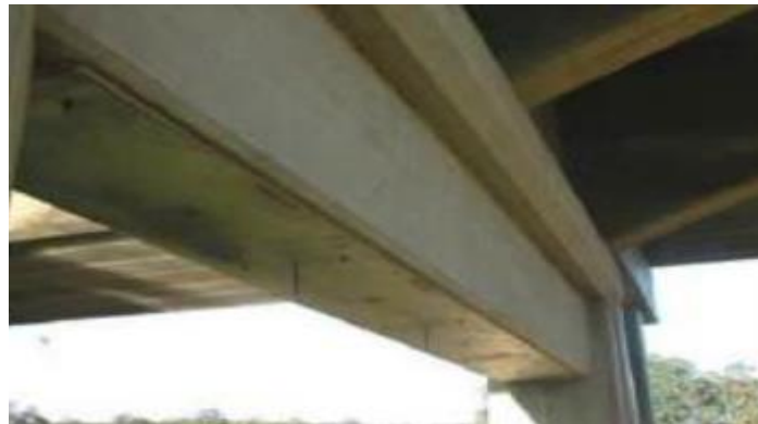
Figure 6 External Steel Plate
