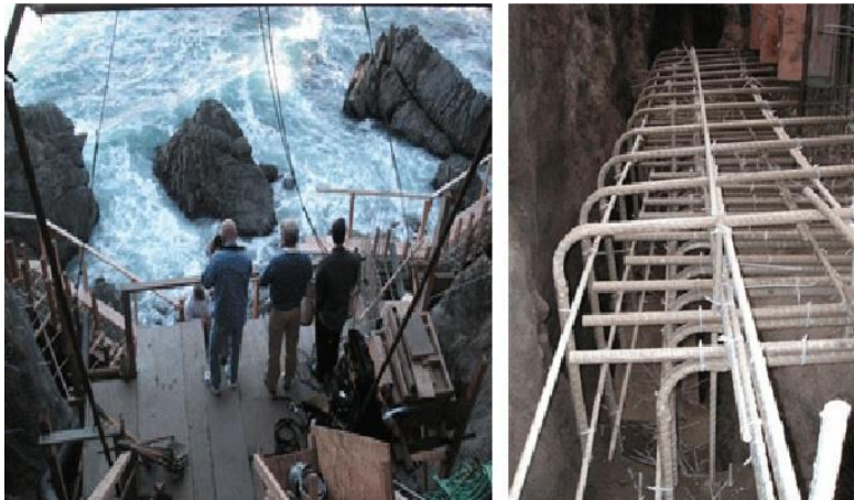
Figure 14 : Seawall of Lyles residence in California, USA (Aslan FRP, 2018)
