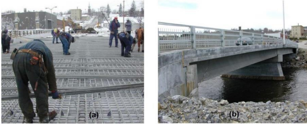
Figure 8: GFRP Bridge Deck, Cookshire-Eaton, Quebec (a) Under construction (b) In service (Muhammad, 2019)
