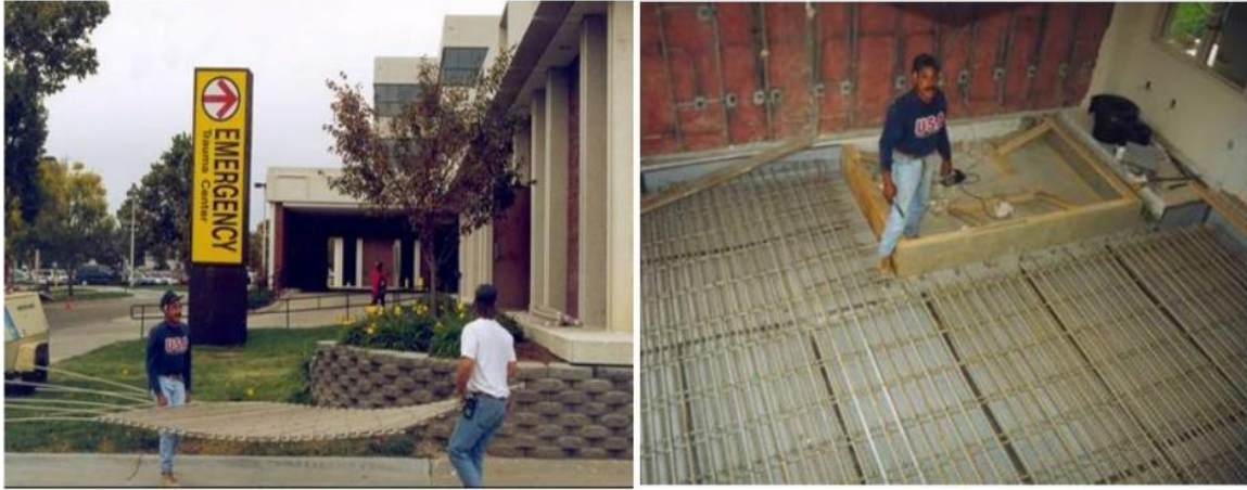
Figure 11 MRI room in Lincoln General Hospital, NE, USA (Aslan FRP, 2022a).
