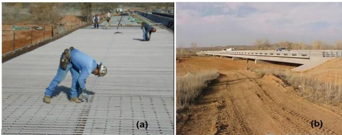
Figure 7 Sierrita de la Cruz Creek Bridge, Potter County, Texas (a) Under construction (b) In service (Salh, n.d.)
