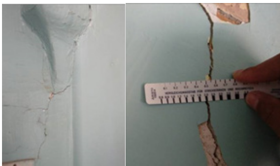
Figure 2. Cracks appeared in the internal plastering la
