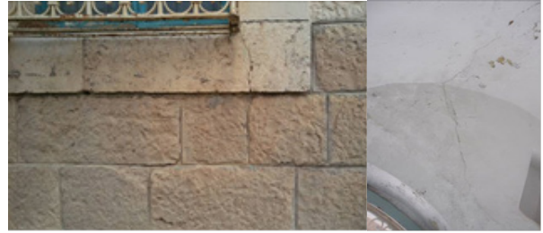
Figure 3. Cracks appeared in the arched opens and in the sill stone at western window open
