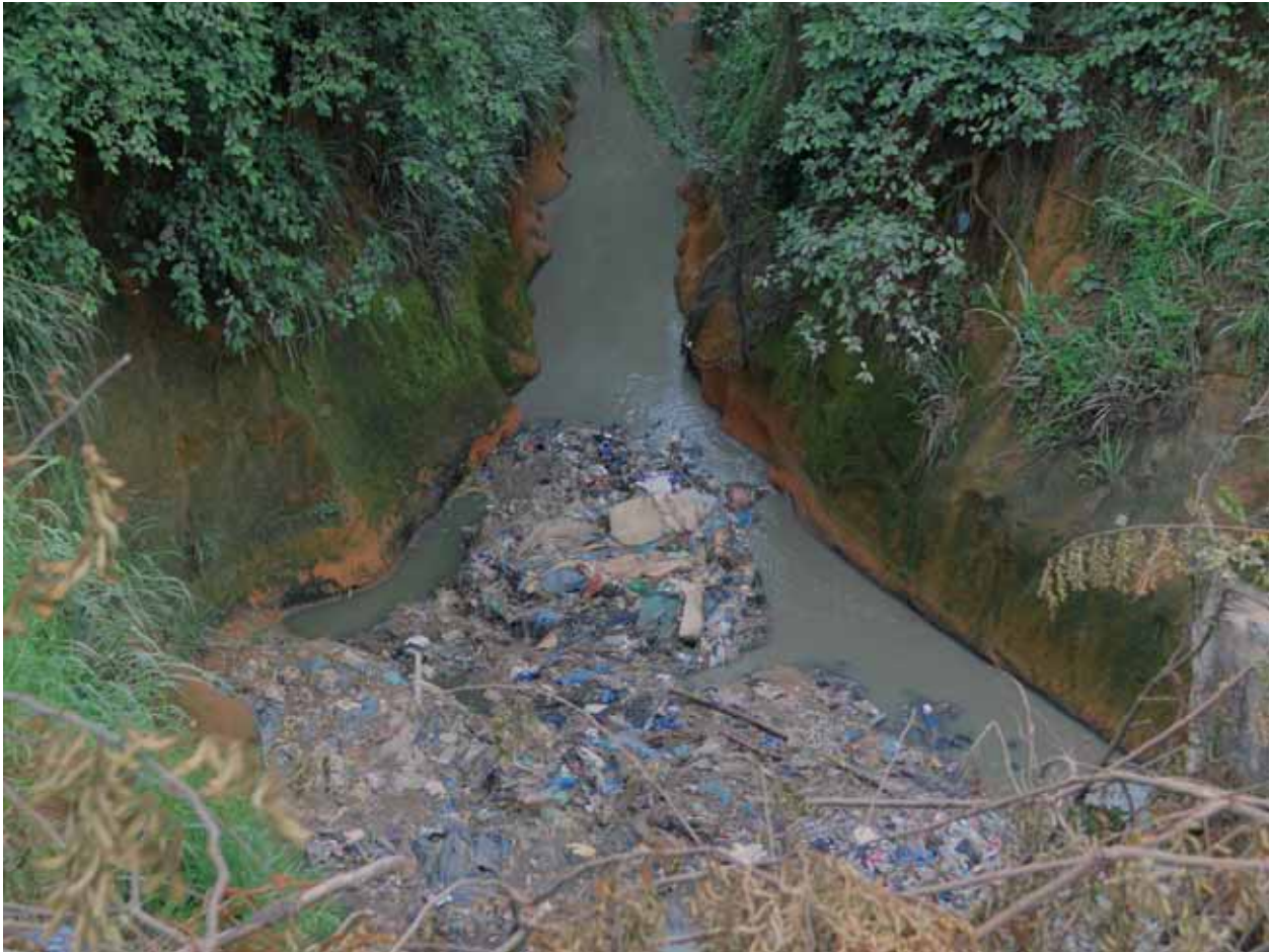
When proper sewage and solid waste management system are absent, gullies get filled with both
