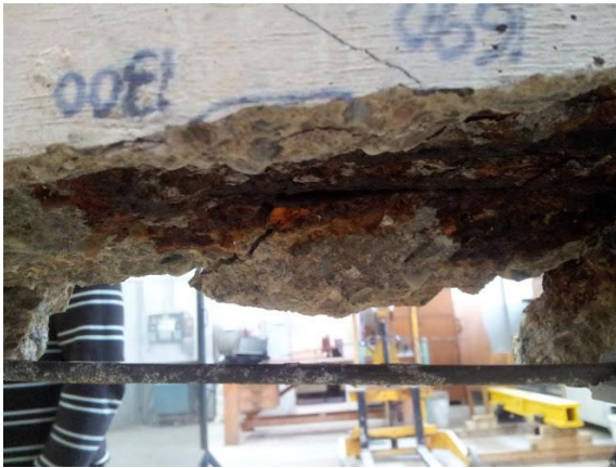
a) A1CL3-R Corroded Beam
