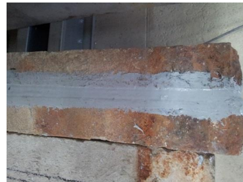
b) A1CL3-R Corroded Beam
