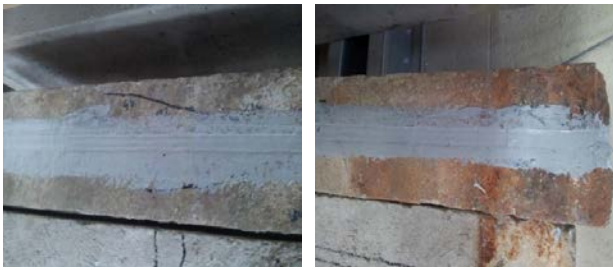
a. A1T Control Beam b. A1CL3 Corroded Beam
