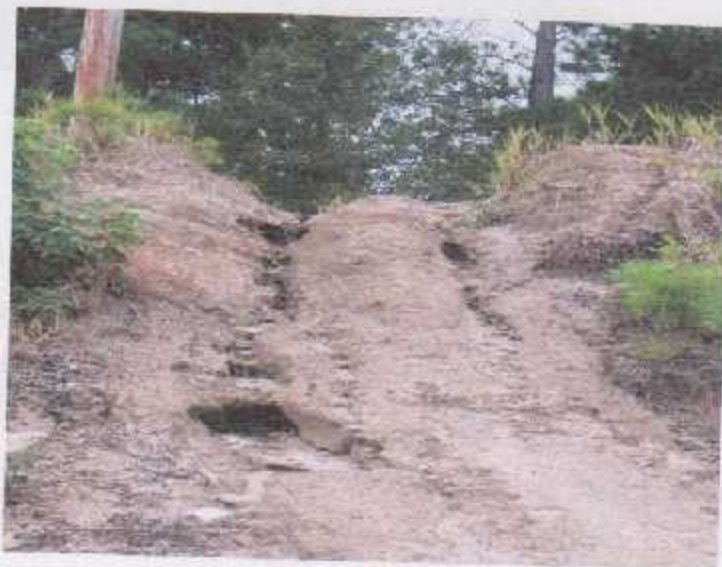
Figure (3.1): Erosion sample, ref (7).
