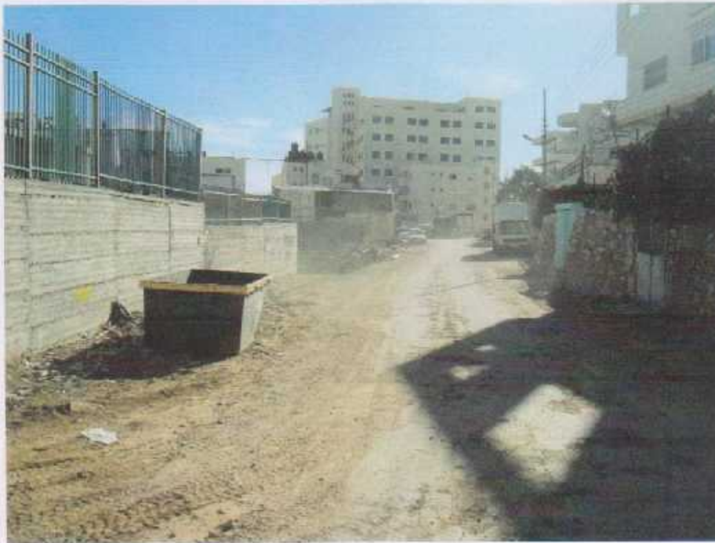
Figure 6-1: Damaged streets near industrial areas Source: researchers lens
