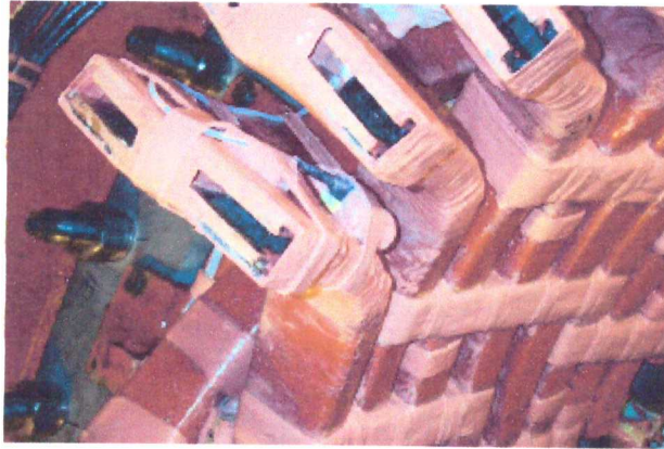
Figure (1.2) Installation of the sensor head and optical cable to brace end-windings
