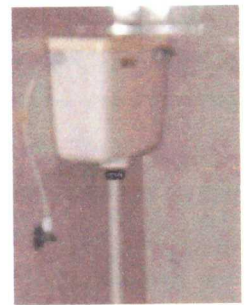
Figure (3 – 10): Flush tank
