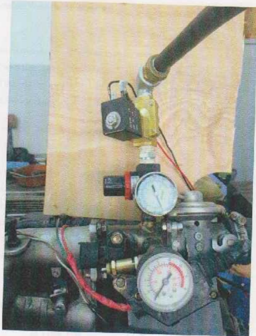
Figure 6.6 Pressure regulator and Solenoid valve
