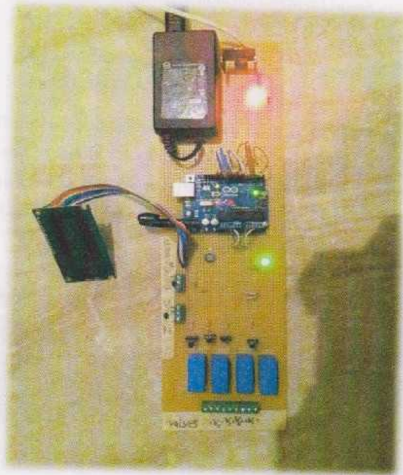
Figure (4.5): Control Panel
