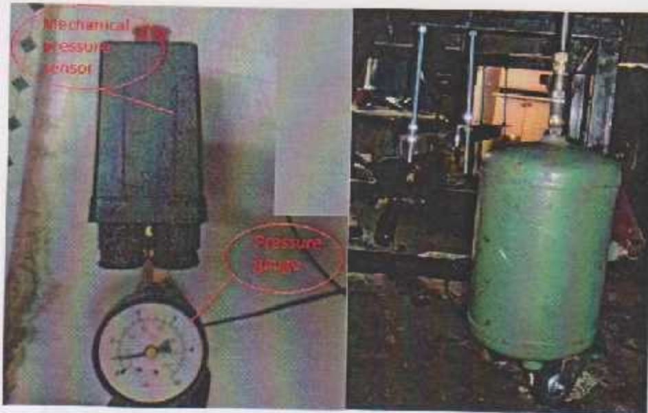
Figure (5-7) shows the used air tank and mechanical pressure sensor
