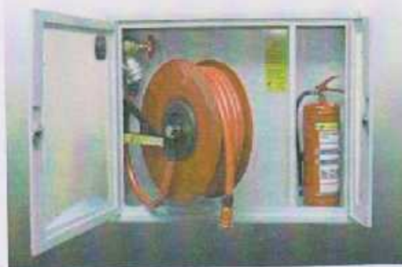
Figure (4.3): Fire hose cabinet
