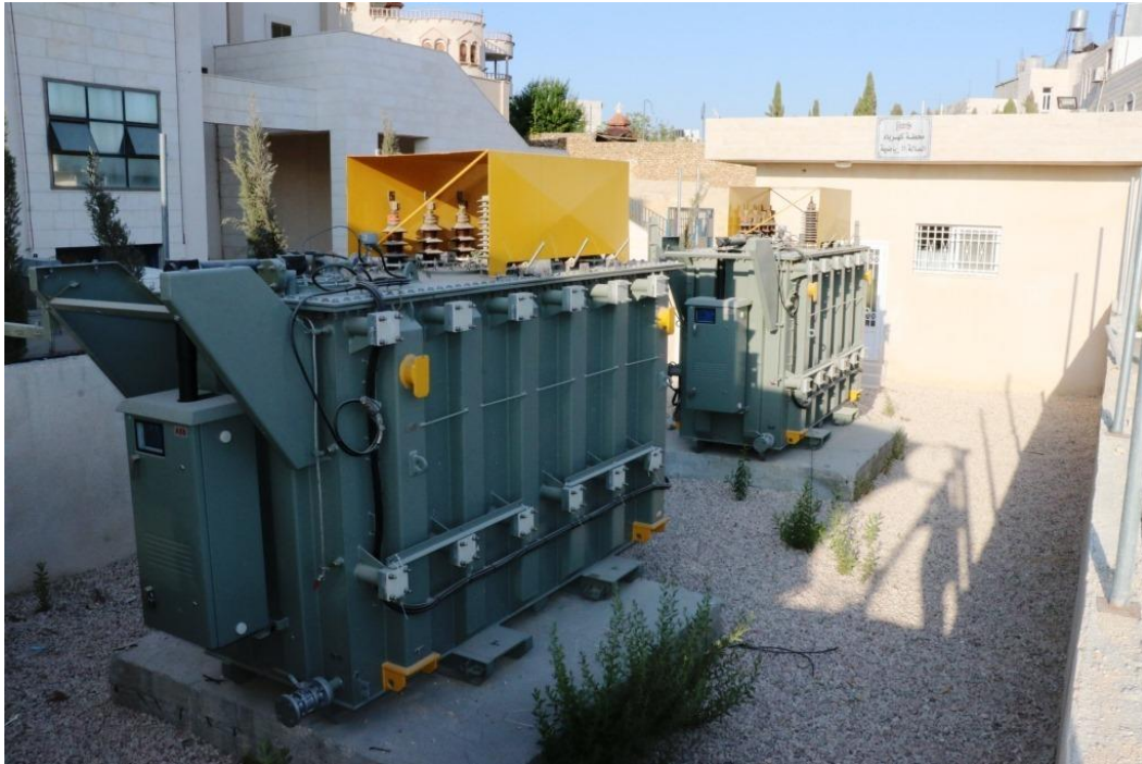
Figure 2. 12:New MV Substation .
