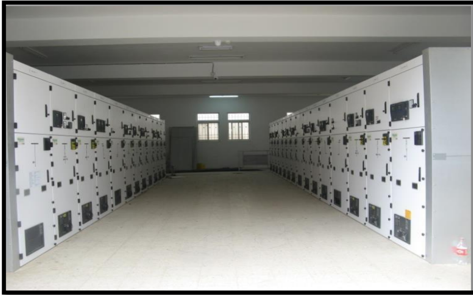
Figure 2. 3: Main Power Center .
