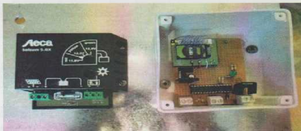
Figure 5.19: GSM and Charge Controller After Fixed Both on the Panel
