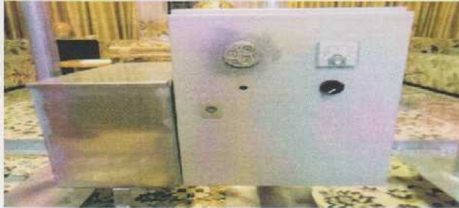
Figure 5.20: Electrical Switch Board
