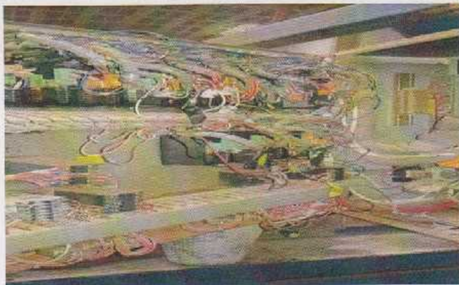
Figure (6.11): The connection inside the control panel.
