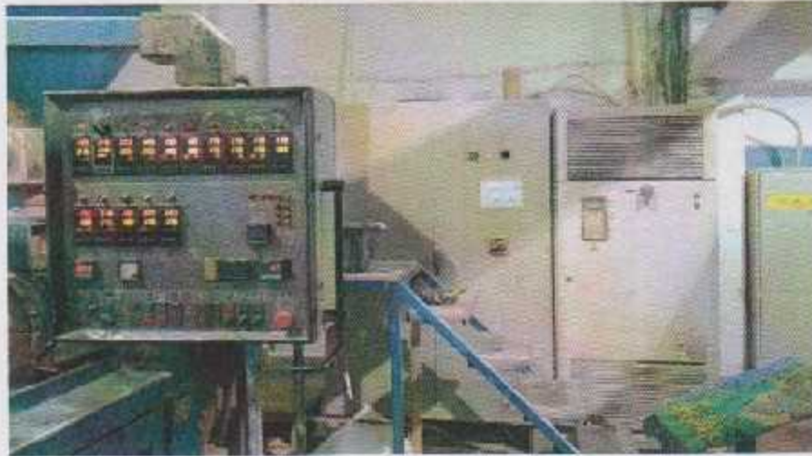
Figure (6.10): The old control panel.
