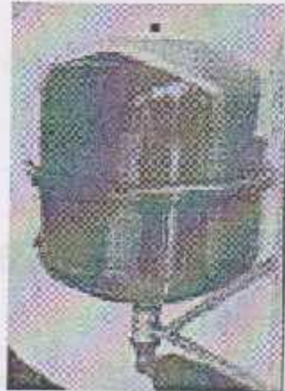
Fig 2.6 Close expansion tank
