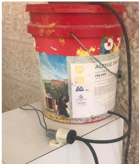
Figure 5.4: Pump 2 connected with water tank to the field
