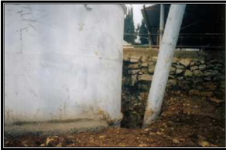
Figure A-5: Digester + connection pipe to the outlet chamber.
