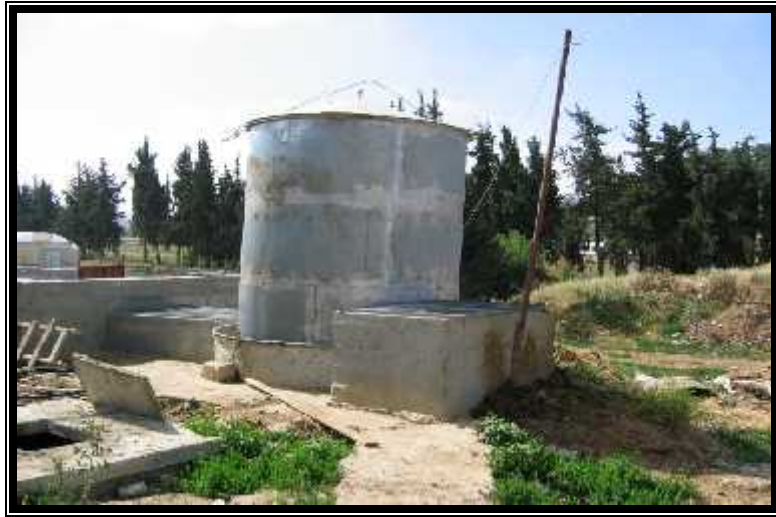
Figure A-19: Gas holder full of biogas
