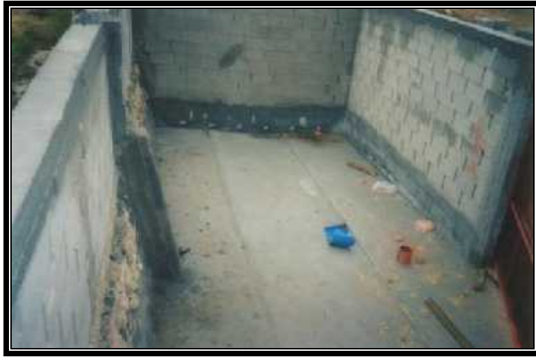
Figure A-4: Composting facility (chamber receiving the biogas slurry)
