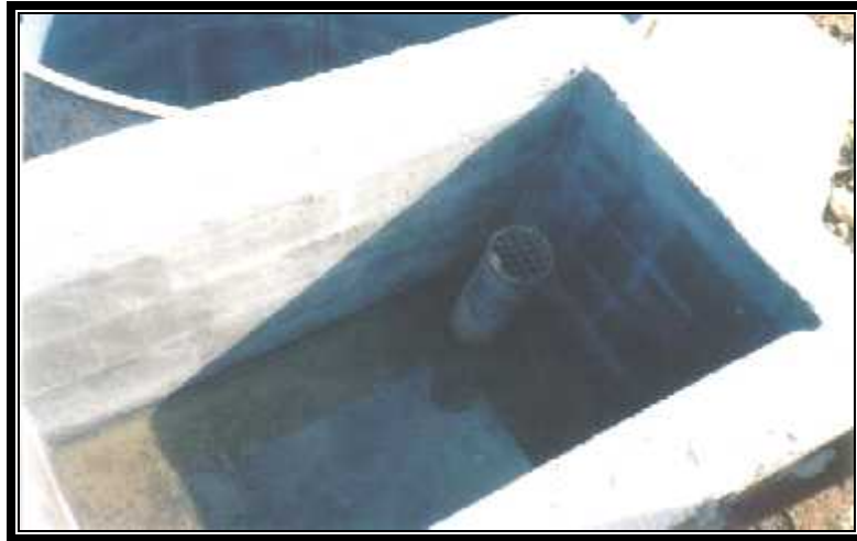
Figure A-10: Inlet pipe 6" in the mixing chamber with screened mesh (notice that the pipe is 30cm higher than the ground).
