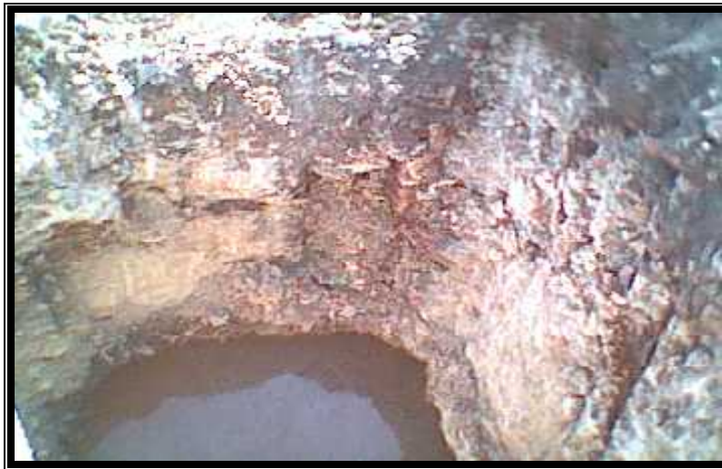
Figure A-2: The pit dug for the AFC plant, rain water was emptied afterwards.
