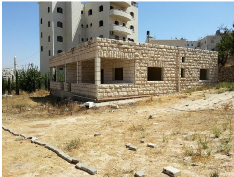
Figure(5.4)photo for the house that would be built 3D model to it
