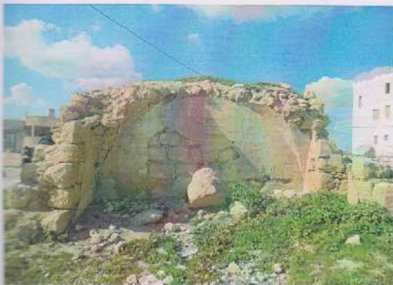
Figure (2.28): Buildings in poor condition [ Project Team ].
