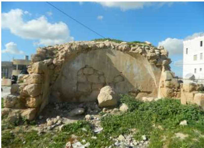
Figure (2.28): Buildings in poor condition [ Project Team ].
