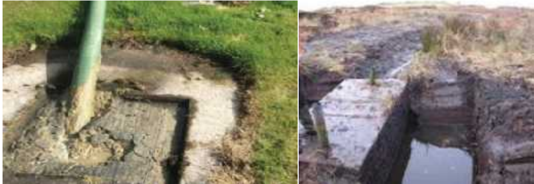
Figure (4.2): Collapse of Septic Tank due to lack of maintenance
