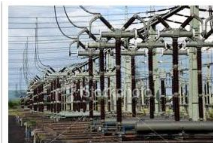
Figure 3.1. View of substation
