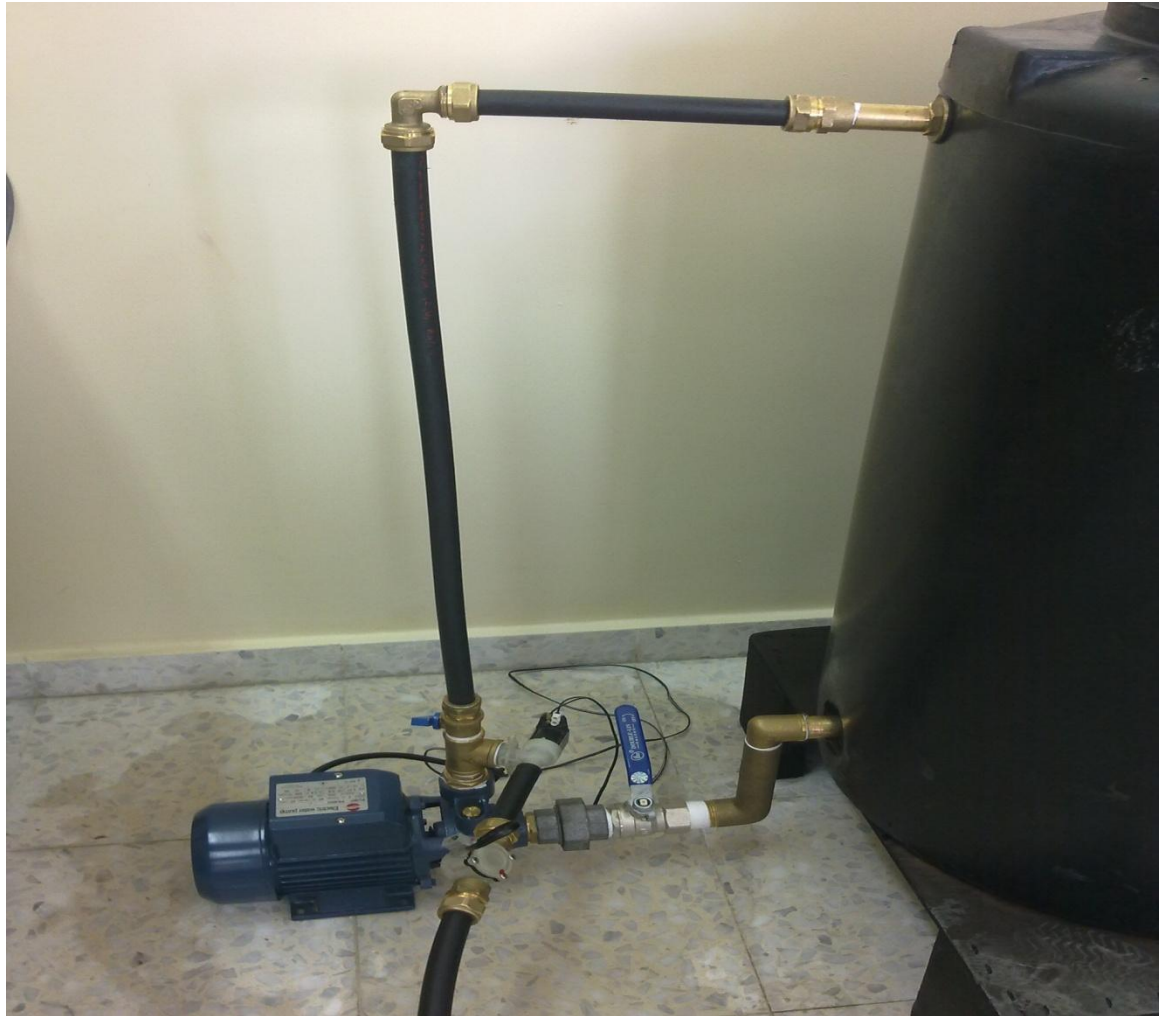
Figure (6.4) The Valve and Pump.
