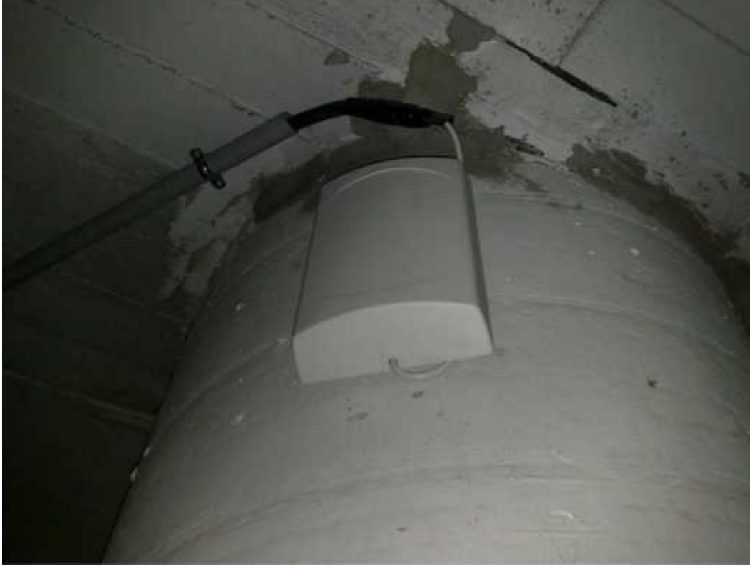
Figure 4.10: Indoor antenna at ground floor in Hebron center
