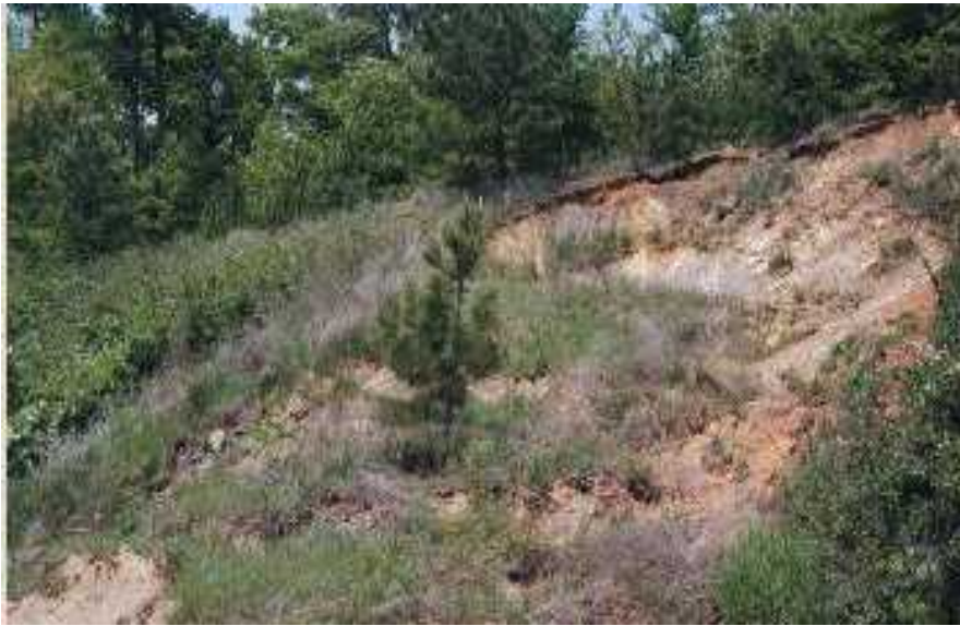
Figure (4.7): Rapid Movement (Slump), (Reference 10)
