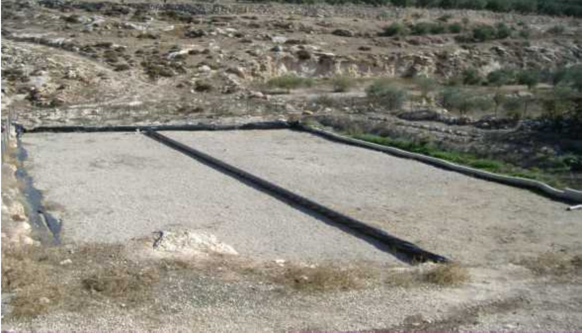
Fig (4.25): Wet Land at Nuba Wastewater Treatment Plant
