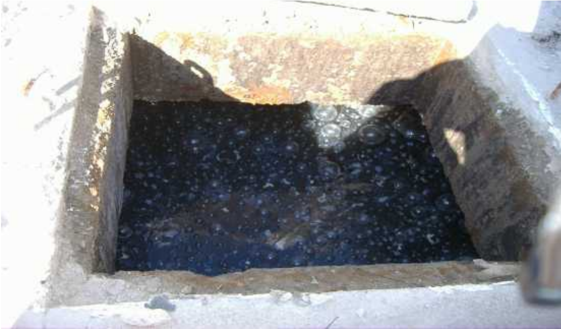
Fig (B.15): Septic Tank with Methane Gas Bubble
