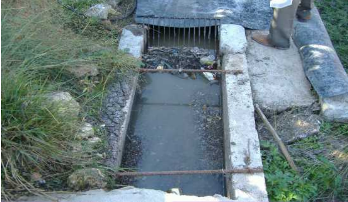
Fig (B.19): Wastewater Treatment by Bar Screen
