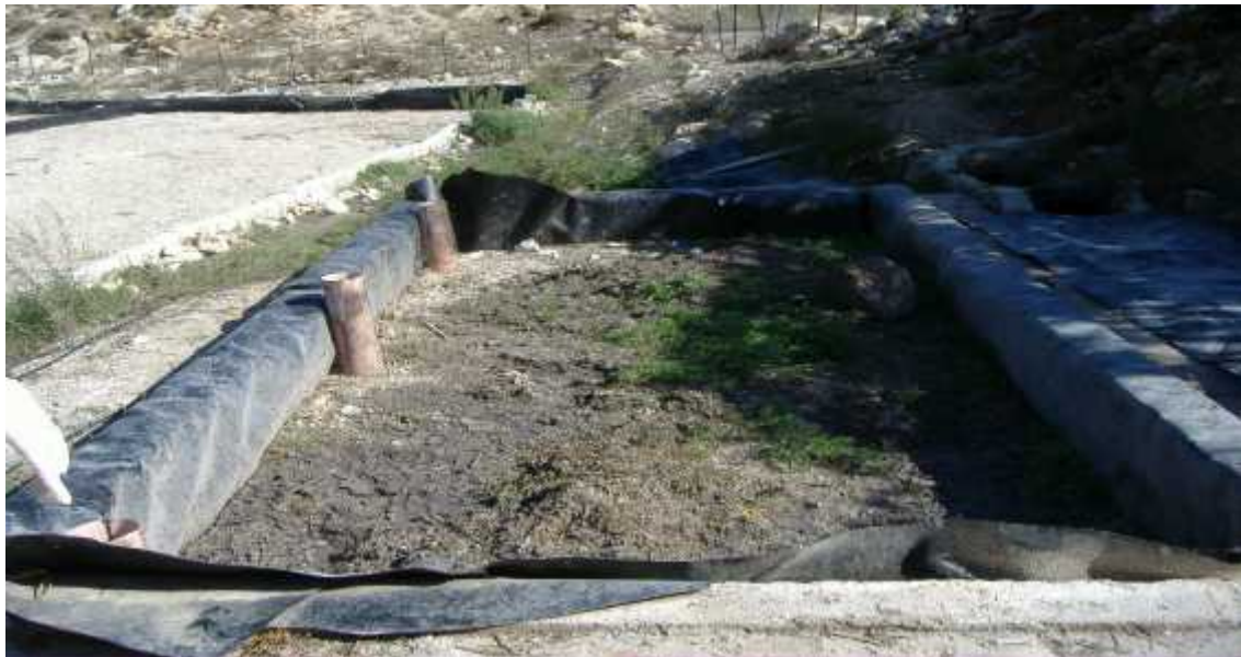
Fig (B.22): Sludge Bed at Nuba WWTP
