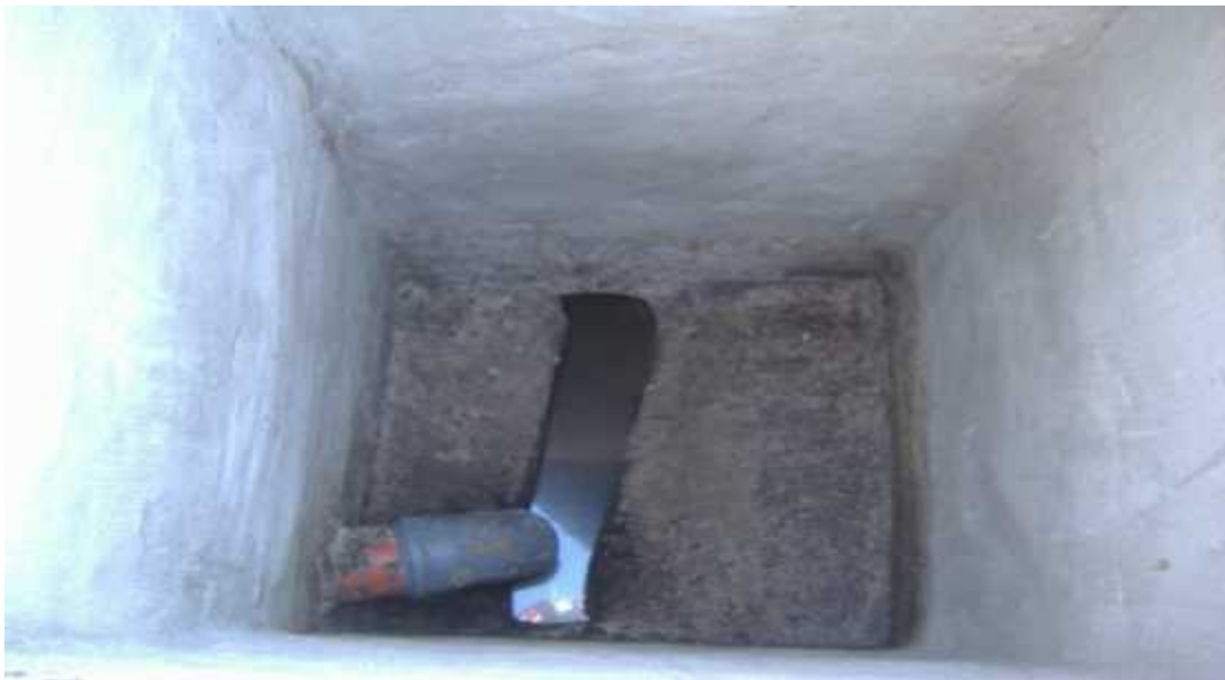
Fig (4.18): Top View of the Storage Tank
