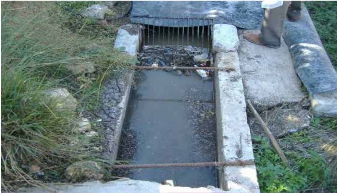
Fig. (4.21): Bar Screen Photo in the Treatment Plant
