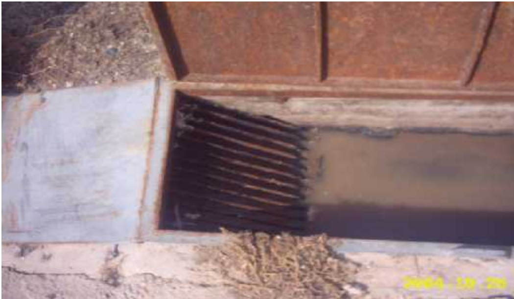
Fig (B.2): Bar Screen and Channel
