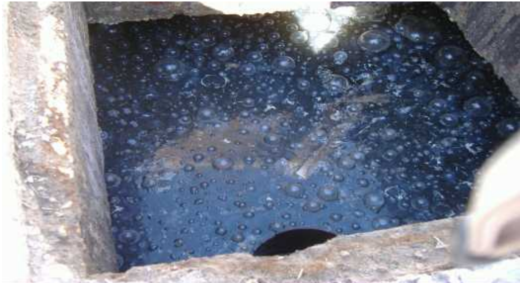
Fig (4.16): Anaerobic Biofilter Opening
