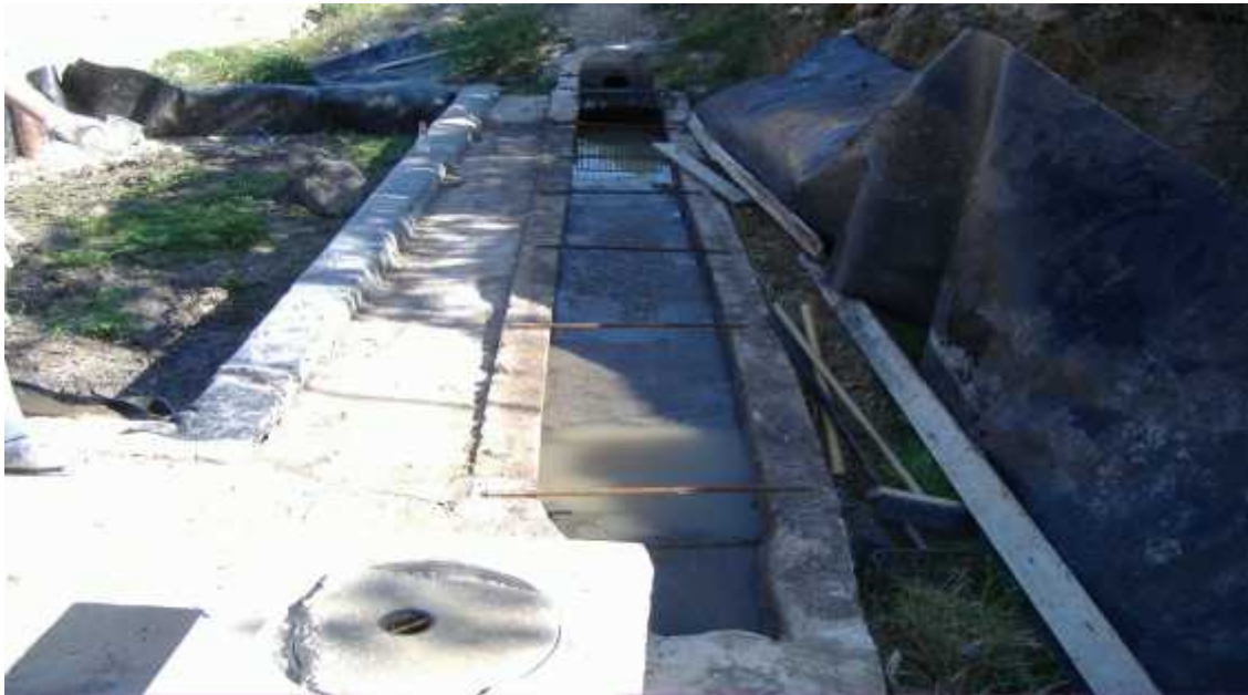
Fig (B.18): Screening and Channel at Nuba WWTP
