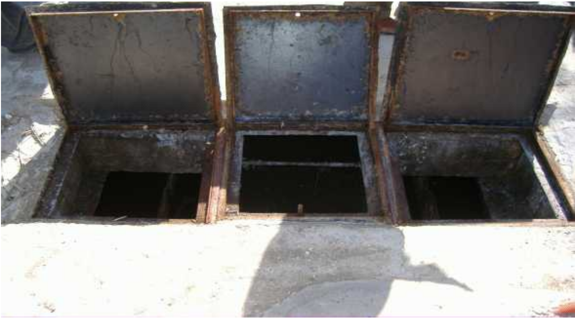
Fig (4.23): UASB Storage Tanks
