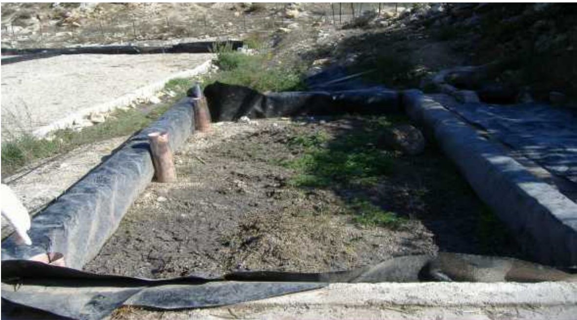
Fig (4.24): Sludge Drying Bed
