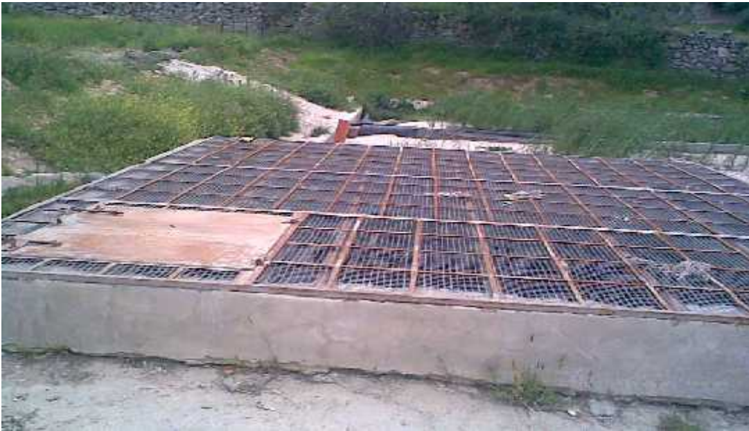
Fig (B.8): Treated Wastewater Storage Tank
