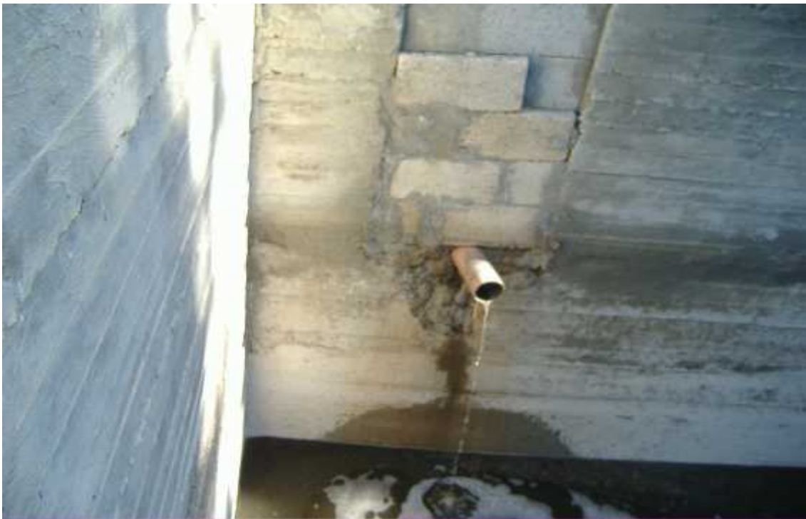
Fig (B.32): Storage Tank at Al Aroub WWTP
