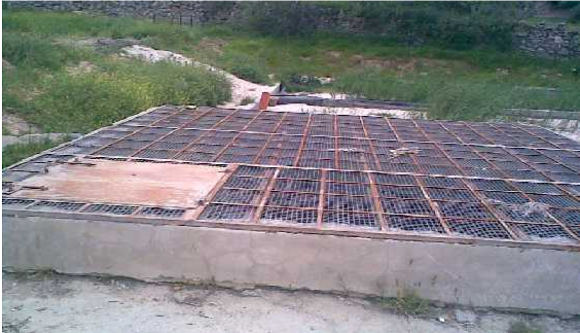
Fig (4.9): Picture of the Storage Tank
