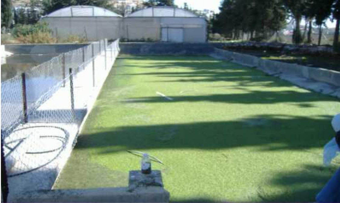
Fig (4.33): Duckweed Ponds at Al Aroub Wastewater Treatment Plant
