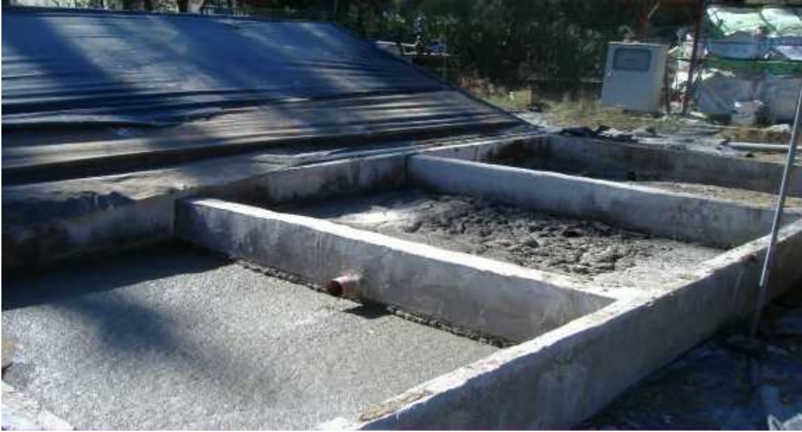
Fig (4.31): Settling Tanks at Al Aroub Wastewater Treatment Plant
