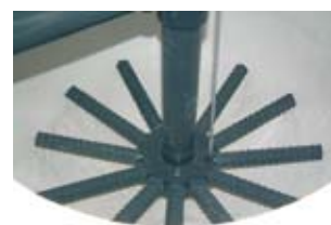
Collector arms detail
