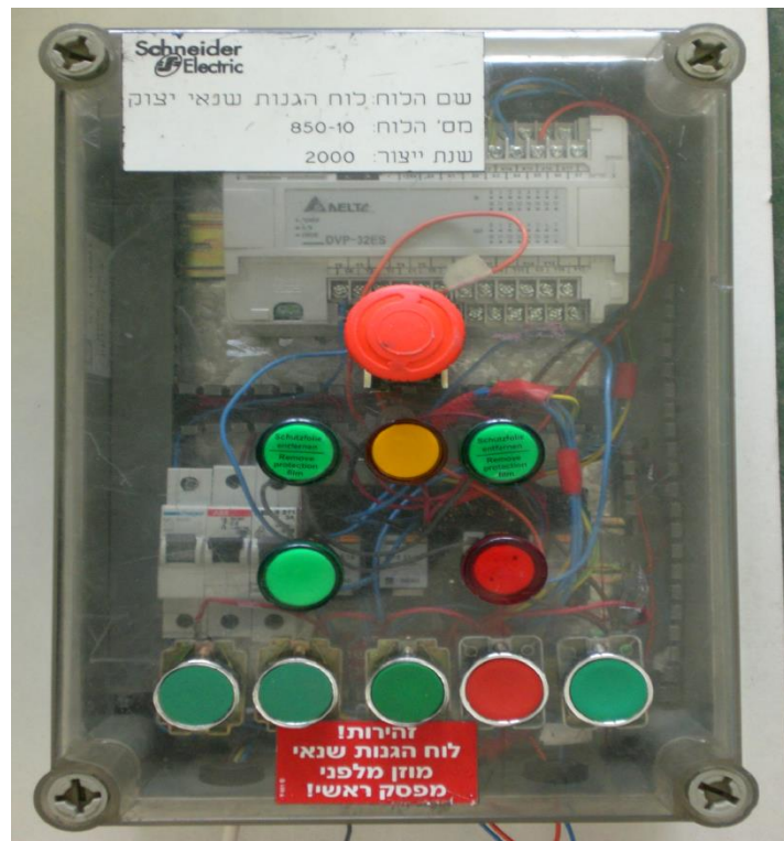
Figure 4.6 Box contain PLC and other hardware for the System
