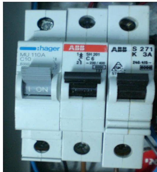
Figure 4.5 Circuit breaker for the System
