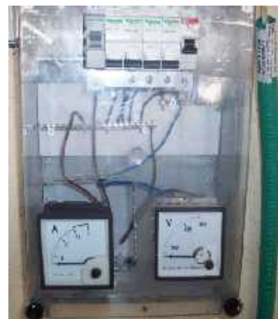
Figure 3.16: Control Load Unit
